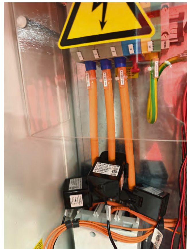
3 phase current clamps from Pressac Communications installed on the CNC machine's incoming mains.
